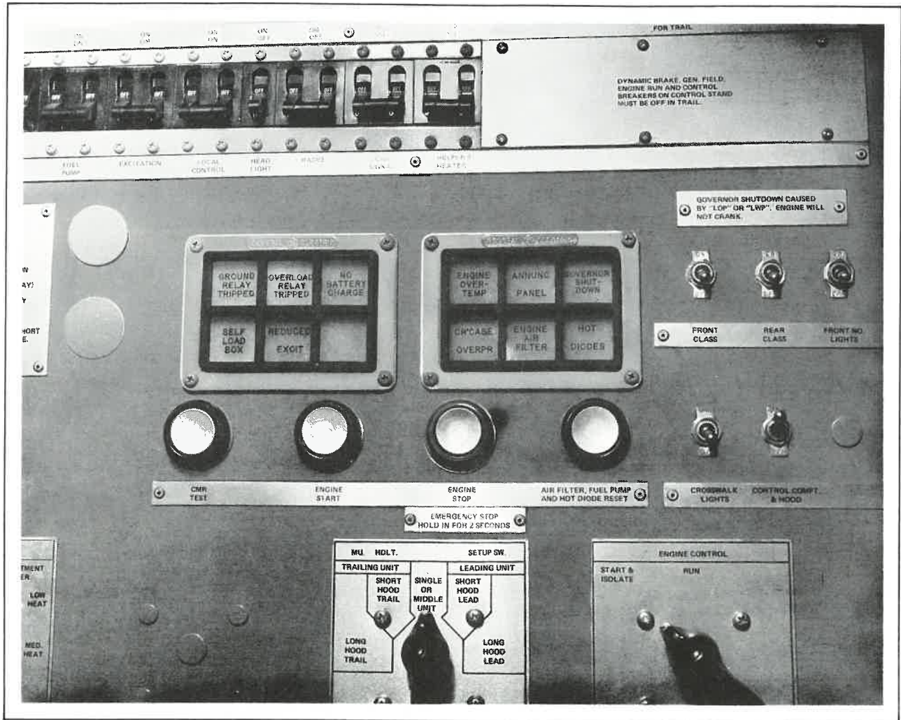
FIG. VIII-18. ENGINE CONTROL PANEL INDICATING LIGHTS.
