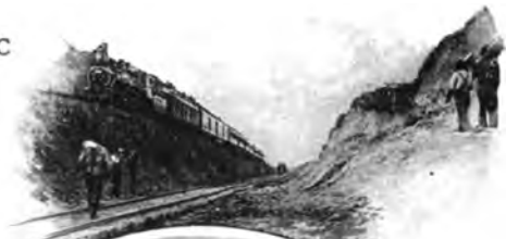
Reducing a Grade. Last Train over OLD Main Line. New Track Been in Cut before Leveling, etc.
