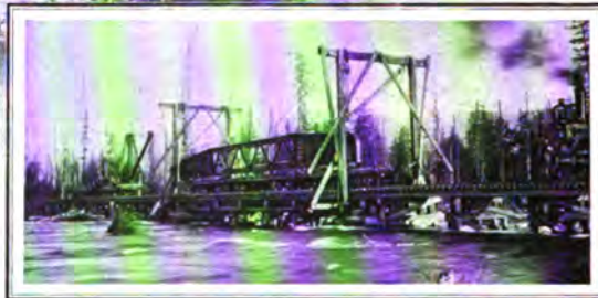
Raised from Cars by Locomotive at one end and by Hoisting Engine at other. Note Position of Tackle.
